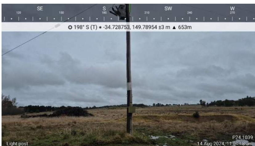
Photograph 6-4 Power Pole with transformer between service shed and cottage
